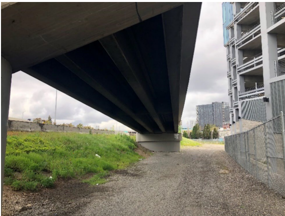
Area C, I-5 ramp with gravel road, fill berm, utilities, and adjacent building, facing north
