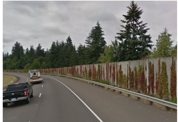
Example sound wall. Sound walls reduce noise for neighborhoods, students, and businesses.
