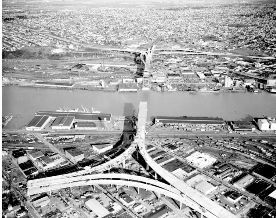
Figure 19. Construction of the Fremont Bridge in 1971, looking east. Courtesy City of Portland Archives.
