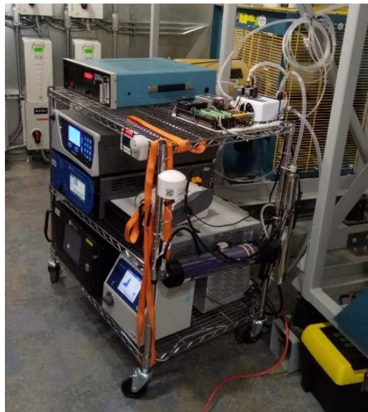
Figure 5b. Installation of a second set of instruments in the AHU-5 at Harriet Tubman Middle School. The instruments deployed here are the same as the instruments of figure 5a. Note that this collection of instrumentation included a switching valve system that enabled measurements to be made in both the supply air and outdoor air.
