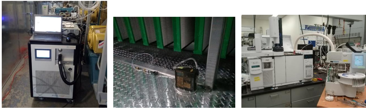
Figure 5c. Volatile Organic Compound (VOCs) monitoring systems. The PTR-TOF-MS (picture on the left) in AHU-5 and sampler and sorbent tubes for GC-MS (picture in the middle) in AHU-3 (pre carbon filter) at Harriet Tubman Middle School. TD-GC-MS in the lab at PSU for the analysis of sorbent tubes (picture on the right).
