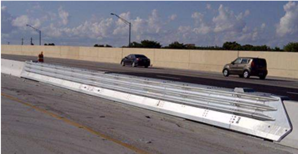
Figure 19 I-87/287 Mario Cuomo Bridge de-mountable barrier, NY
